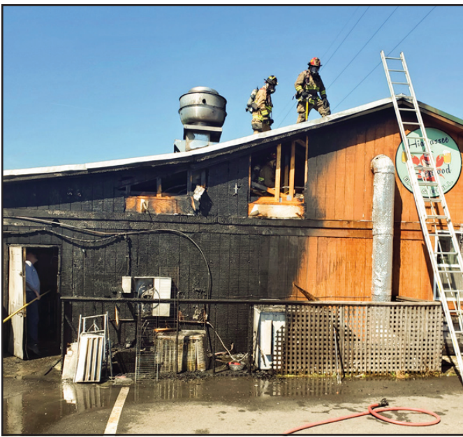
Towns County Firefighters responded to the Hiawassee Seafood fire within two minutes Friday, allowing for a quick knockdown of the blaze before it could destroy the entire building.
